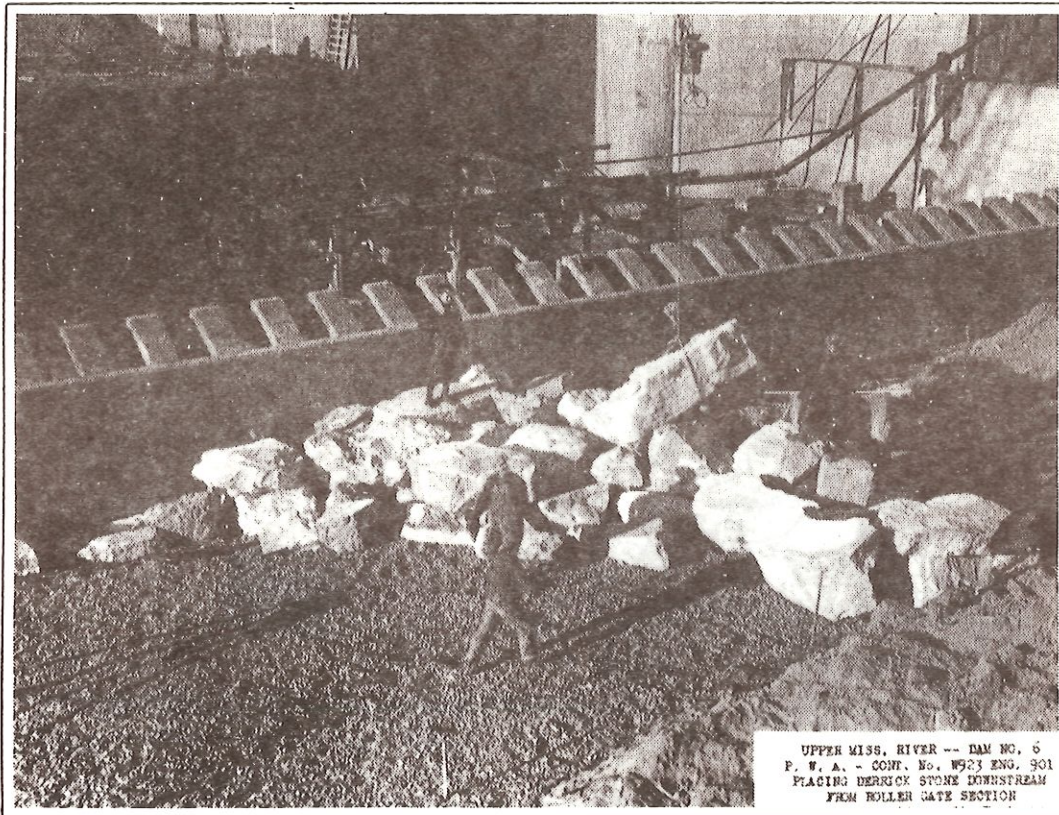
Figure 6 - Placing derrick stone downstream from roller gate section of dam. December, 1935. Corps of Engineers photo.
